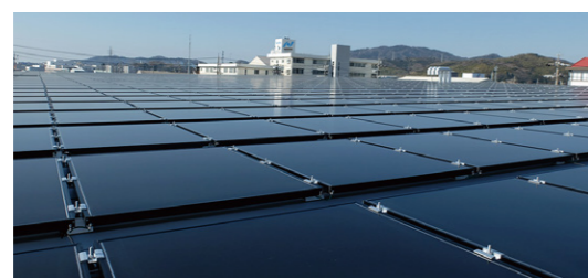
Solar panel of Hiroishi Plant Building 7
